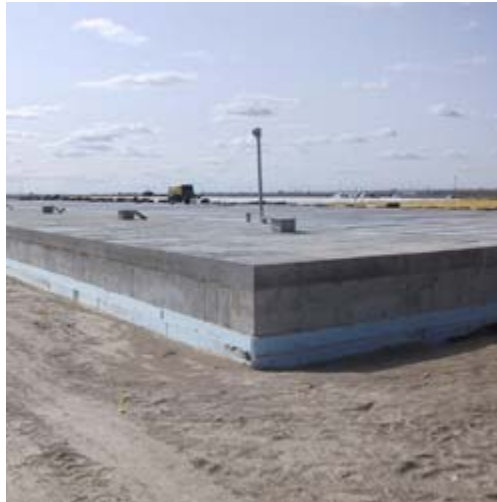
This is the anaerobic digester in Dry Creek, Idaho.
